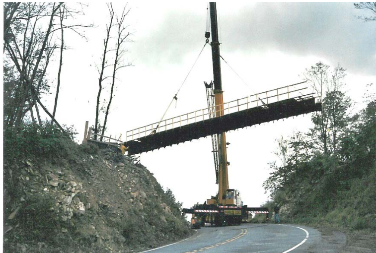
Thanks go to Richard Martin for this photo of the Rt. 225 bridge being put into position.
